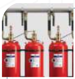
Fire Fighting System
